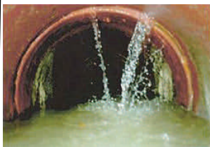
Infiltration in a sewer
