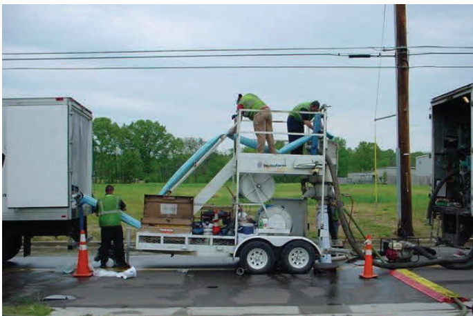
A resin impregnated felt liner is pulled or inverted into the sewer directly from the truck.
