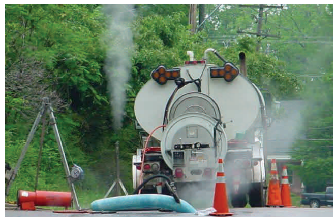
Steam is used to cure the resins in the liner and exhausts out the far end of the liner at a manhole.
